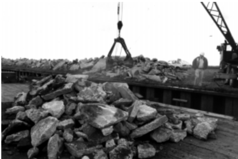
FIGURE 3.—Materials used for construction of artificial reefs at Lorain and Lakewood; reefs consisted of clean concrete, rock, and brick rubble. (Photo courtesy of D. O. Kelch, Ohio Sea Grant.)
