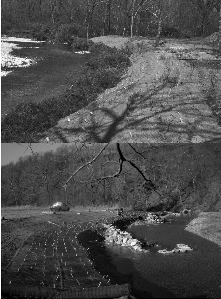
Figure 20.7. Cedar tree revetment (top) used to control streambank erosion and conserve fish habitat in Spring Creek, Oklahoma. J-hook rock vanes (bottom) installed in Honey Creek, Oklahoma, to stabilize streambank erosion and create fish habitat. Erosion control blankets were placed on the streambanks after each project to limit erosion until natural vegetation became reestablished. (Photos by Oklahoma Department of Wildlife Conservation).
